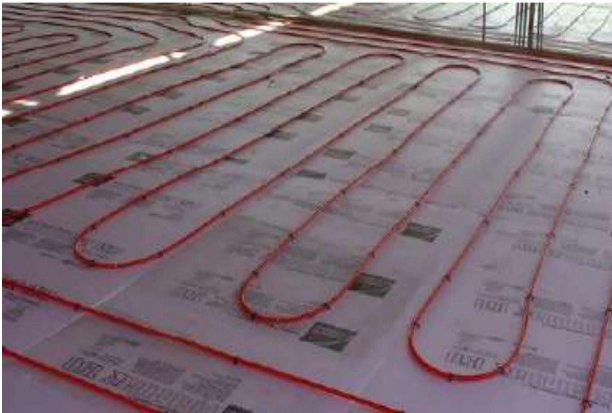
Fig 41: PEX cooling pipes (Vasiliu,2015)
