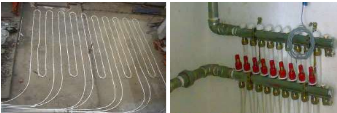
Fig 14: Manifold for PEX cooling pipes, and PEX pipes laid, before pouring of concrete. (Kristensen. P.E & Tang. CK & Reimann. G & Ismail. A.Z, 2008, p.225)
